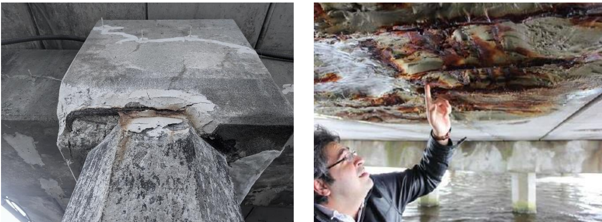
Figure 1. Corroded steel-reinforced concrete structural elements
