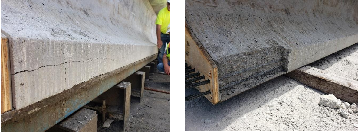
(a) Longitudinal cracks and concrete spalling near the ends
