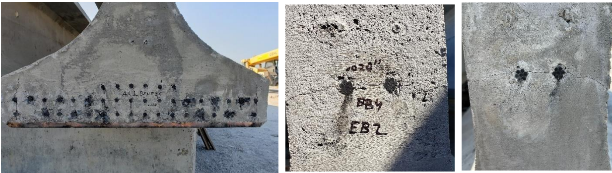
(b) Transverse cracks and strand slippage near the ends
