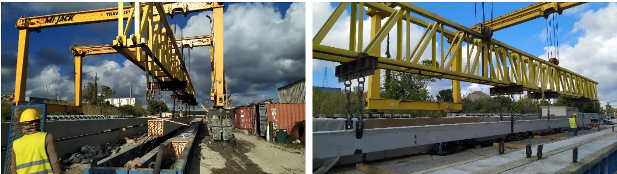
Figure A - 29. Lifting of piles out of their formwork at the precast yard
