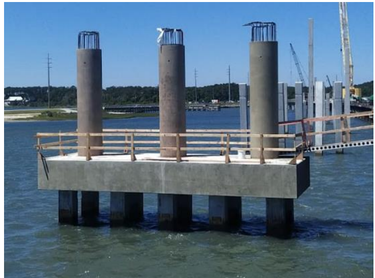
(b) Bent column
