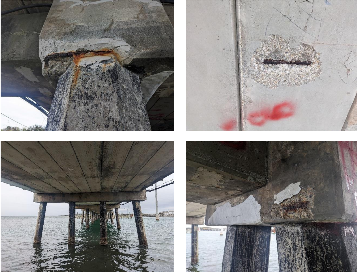
Figure A - 22. Corrosion of existing structural elements
